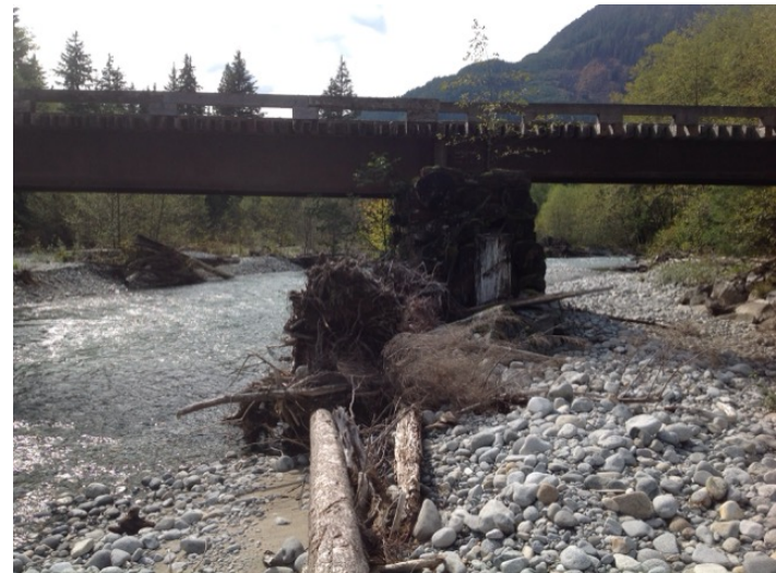
debris accumulation at pier
