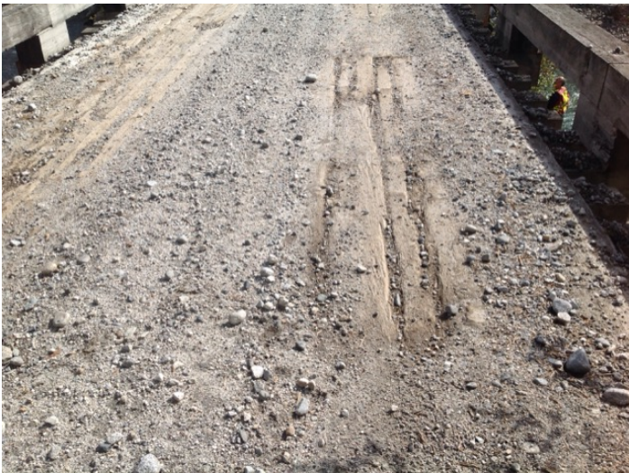
Deck - wear noted on right span on wheel path
